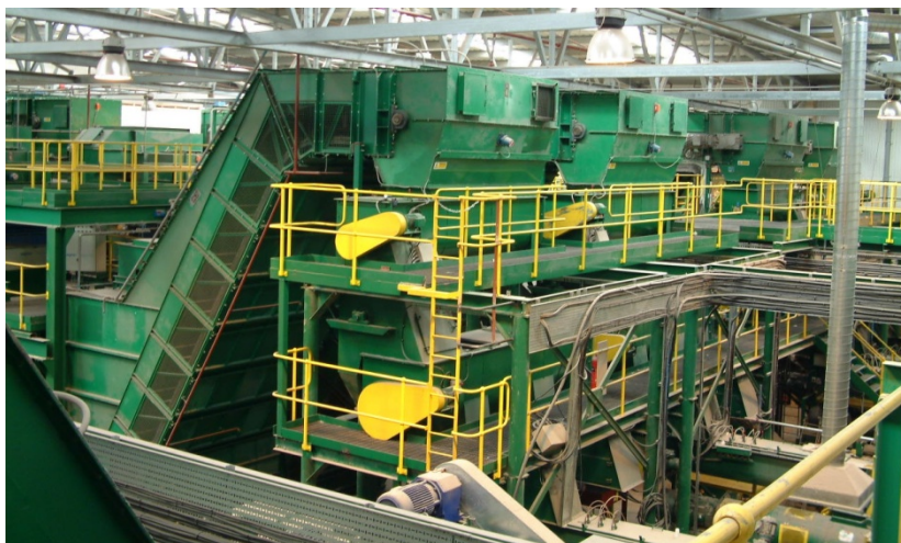
A fuel production plant built by ART in 2003 – processing 230,000 tonnes a year of wastes with no atmospheric emissions.
